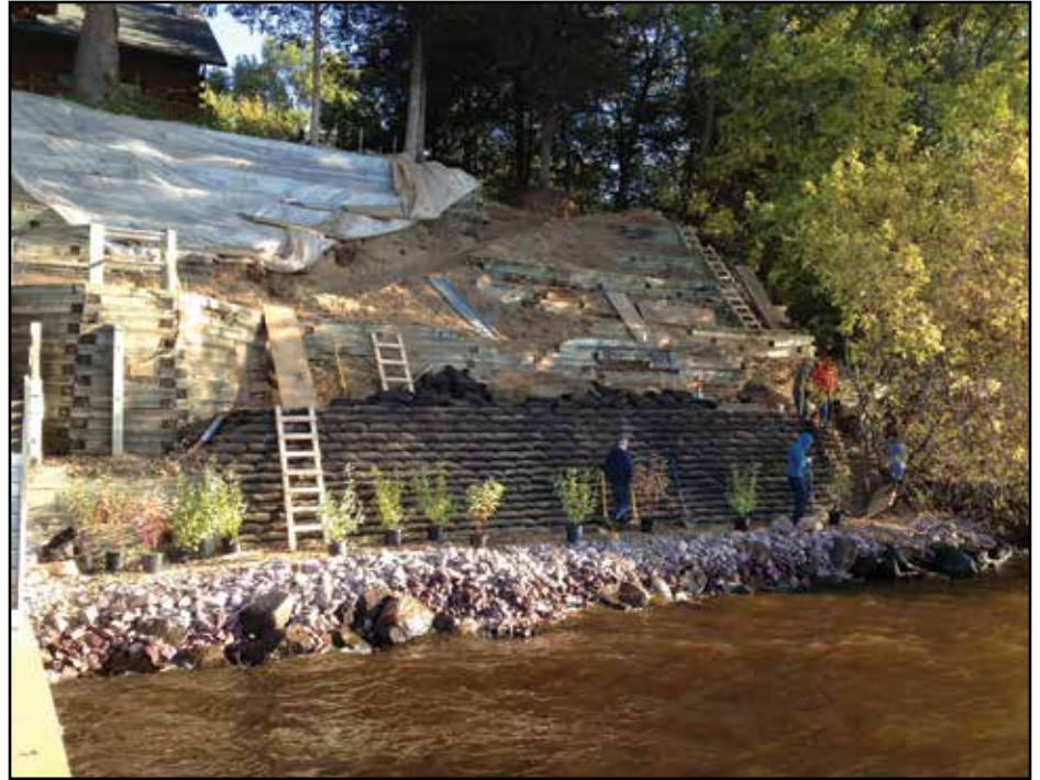
During the fall of 2014, native shrubs were being prepared for planting while soil bag installation was underway.
