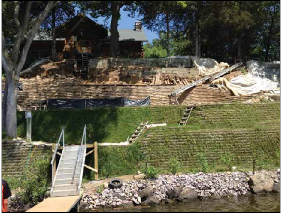
Different stages of the project show the following: vegetated slope on the bottom, constructed wall in the middle, and old existing wall being removed at the top.
